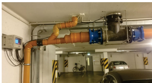
Photo 2. Measurement of stormwater flow rate and the sampling point (phot.: Archive of the Institute of Environmental Engineering and Building Installations)
