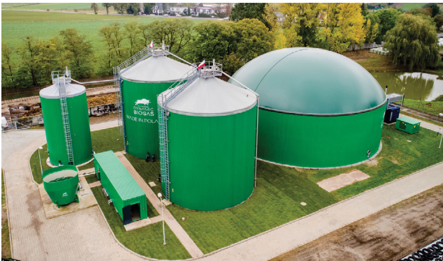
Photo 3. 0.5 MWe biogas plant (Dynamic Biogas technology) with separated acid hydrolysis built in PULS experimental farm in Przybroda in 2019 (phot.: J. Dach)
